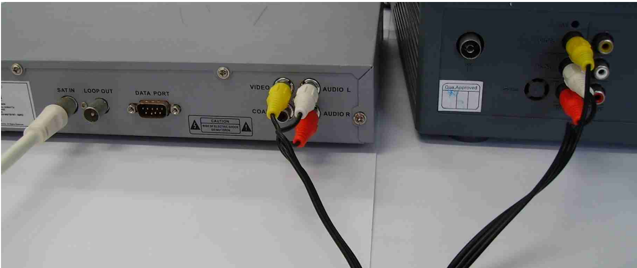
Typical Set Top Box installation without analogue signal bypass.
