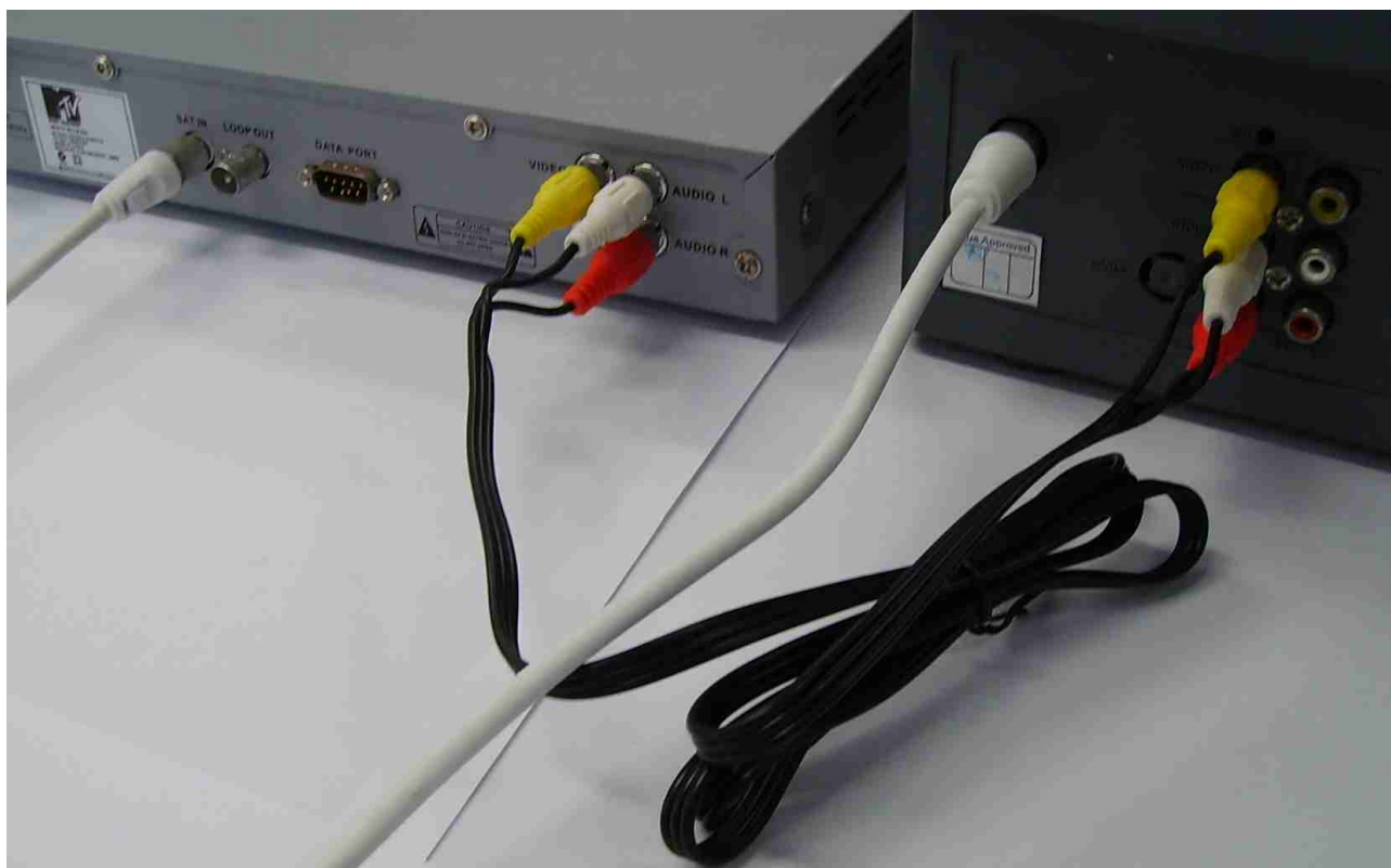
External Set Top Box bypass.
